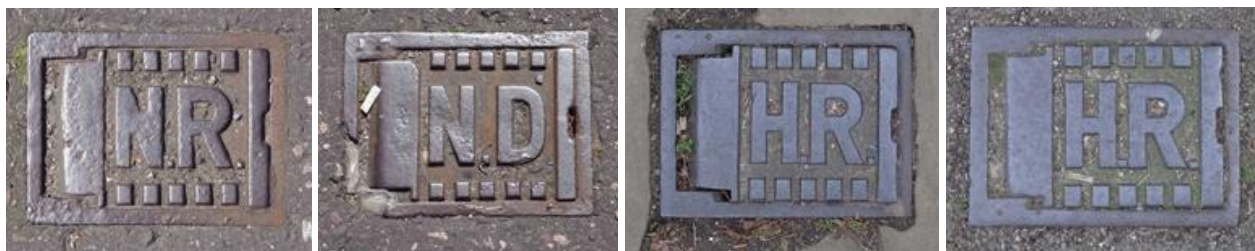
1. N.R. plate, Elsiedene Road N21; 2. N.D. plate, Elsiedene Road N21; 3. H.R. plate, Gordon Road EN2; 4. H.R. plate, Lancaster Road EN2 (footpath to Batley Road)
