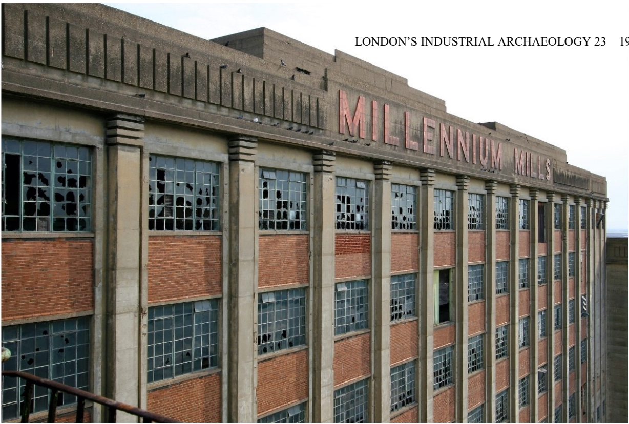
The pediment to the south elevation of Millennium Mills in 2009, which consists of a reinforced concrete dentile course, with the lettering picked out in vitrified red fireclay tiles. This façade was largely hidden until the demolition of the mill's C silo in the 1990s. Picture: Mark Chalmers
